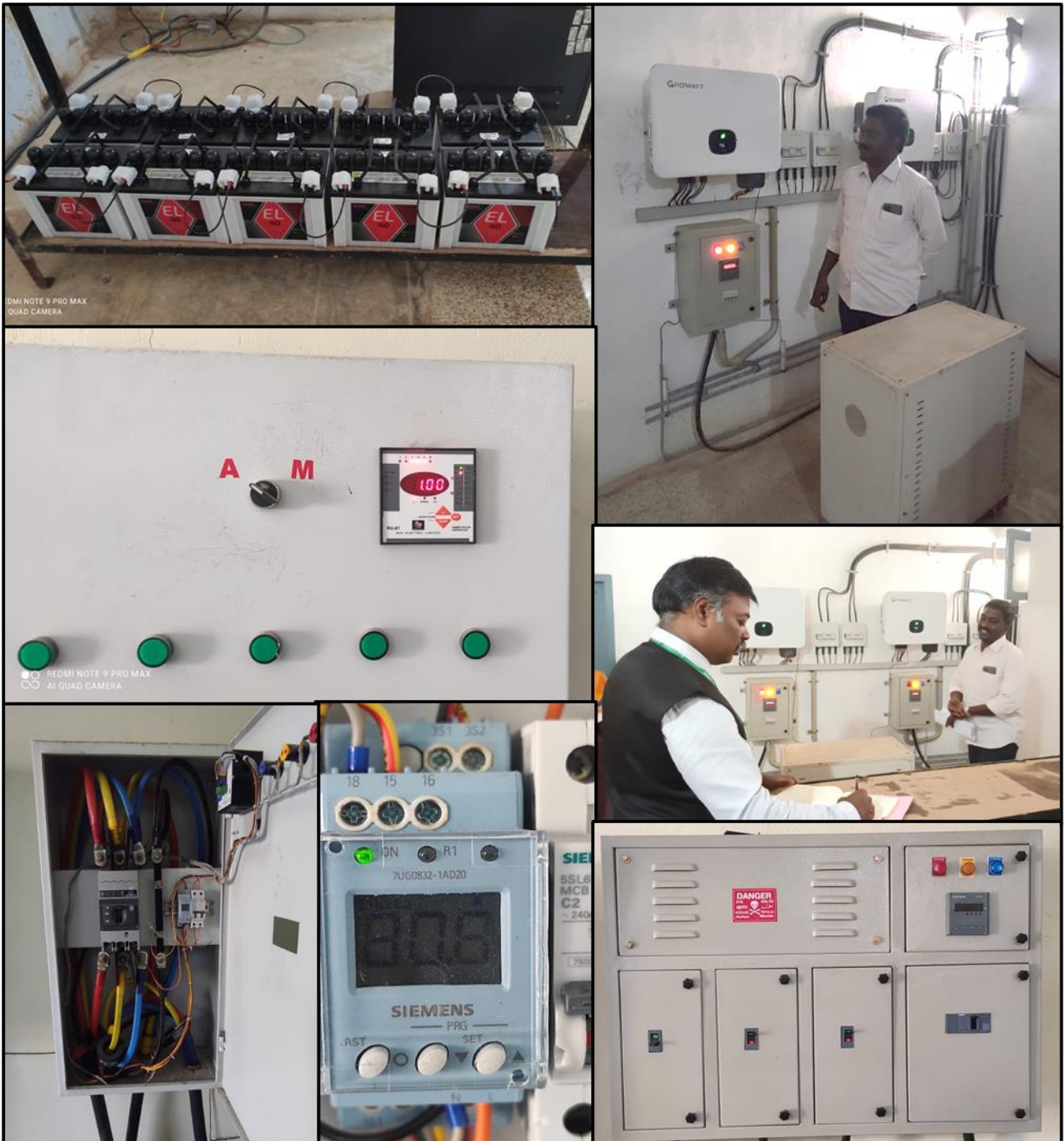
UPS, Generators Facilities Available in Auxilium College (Autonomous), Vellore, Tamil Nadu.
